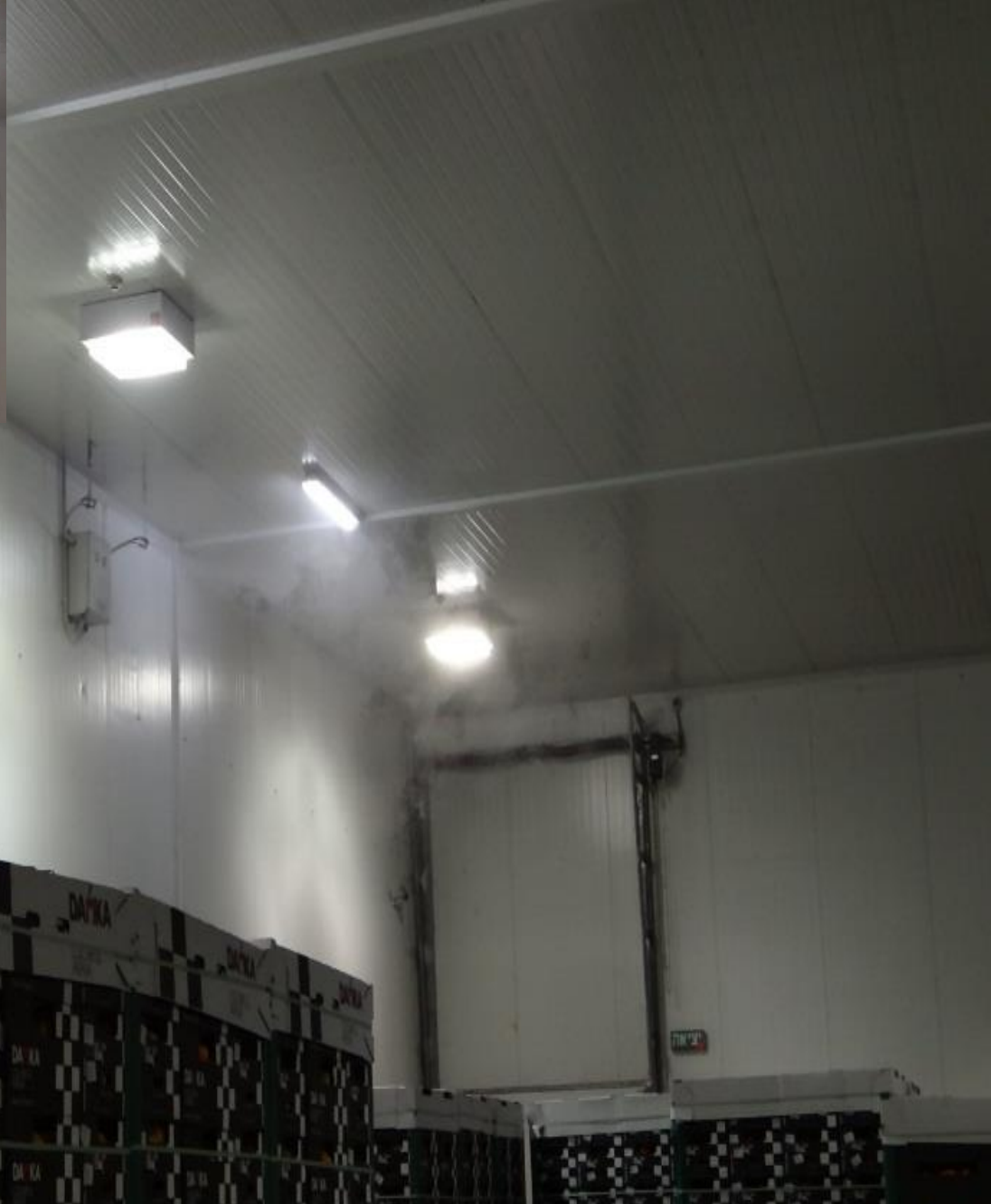
Fog to increase humidity in storage rooms
